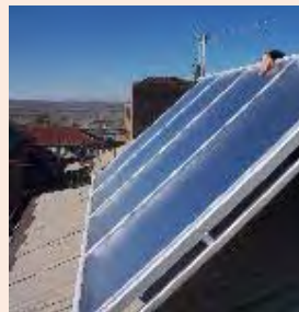
SGP Monitoring visit / Solar collectors installed
